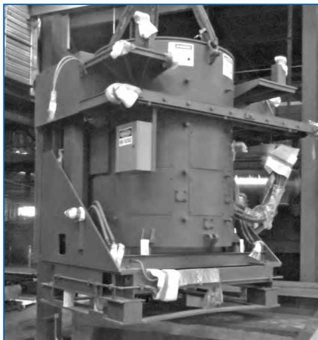
New electric melt furnace installed at Zurn.
