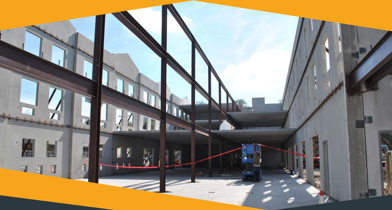
Above: With the walls in place at Metropolitan Ministries' new facility, MiraclePlace, work on the interior infrastructure starts.
