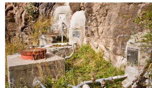
Pueblo of Laguna - Wastewater Treatment System Laguna, NM
