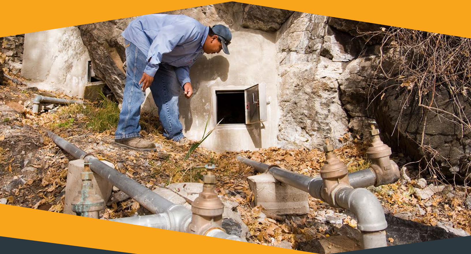
Above: An engineer works on the Pueblo of Laguna water treatment project.
